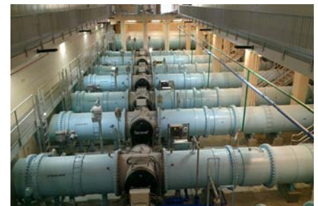
Ultraviolet Disinfection at Miller Treatment Plant
