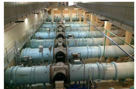
Ultraviolet Disinfection at Miller Treatment Plant
